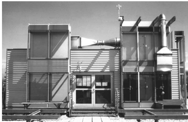
Fig. 2. Outdoor test facility for double-skin-façade systems.
